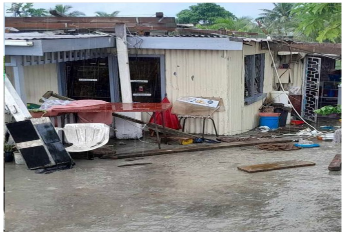
Figure 13b: Damages by mini tornado in Nakasi on the 23 rd . Source: Fijivillage.
